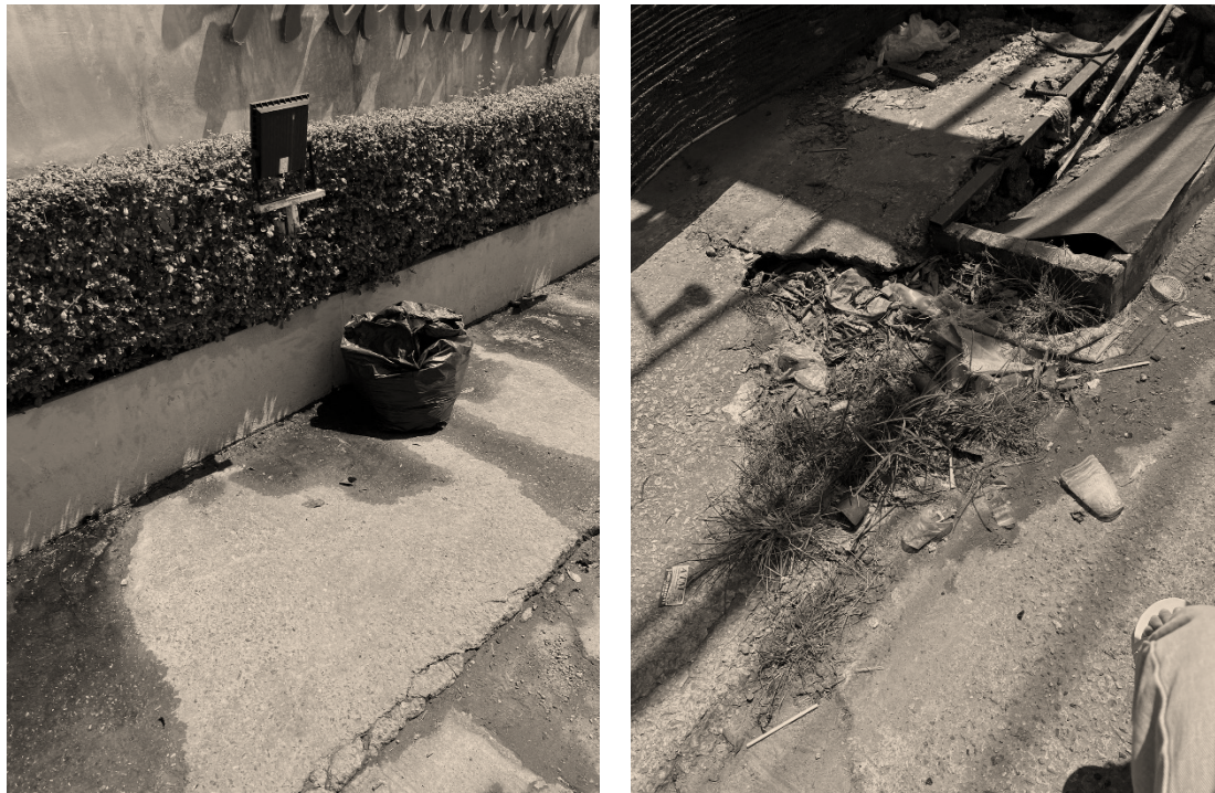
Figure 11. The waste clogged the sewer and the insufficient garbage management Source: data collection by researchers.
