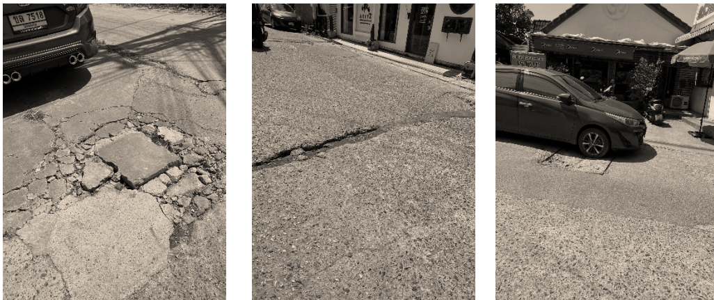
Figure 8. The road surface condition Source: data collection by researchers
